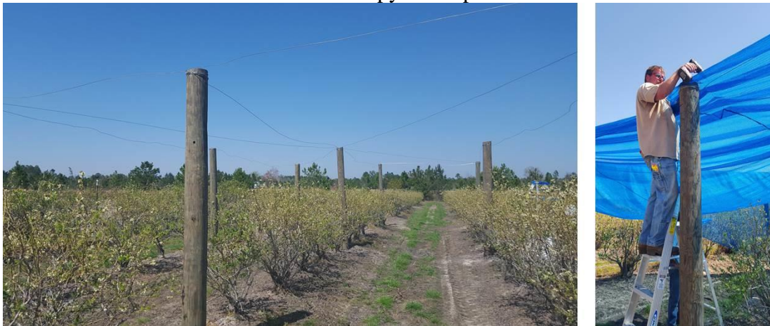
Fig 1. Structural support and the installation of shading nets over ‘Star’ blueberry plants in Alma, GA.
